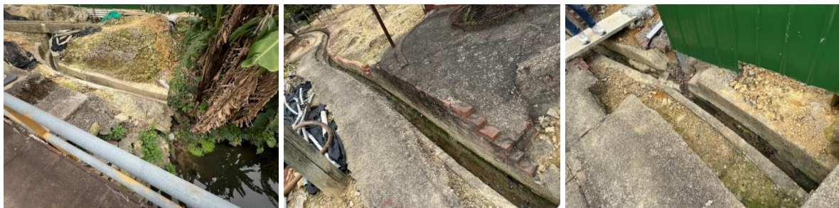
Location and Condition of the Existing U-Channels at West Side (outside the site boundary)
